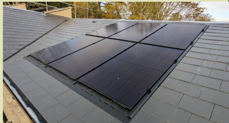
The colour and position of solar panels is carefully defined
